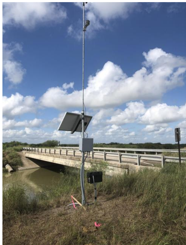
Figure 6. Real time hydrologic system installed in South Texas.
