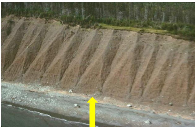
Figure 8. Eroding glacial till cliff with a band of washed off silt-clay sediment (arrow) at the base of the eroding face, Nova Scotia, Canada.
